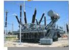
Phase Shifting Transformers
